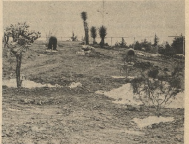
A nature study center is under construction at De Anza. The site, to be completed in June, includes natural terrain from the four California climates of desert, forest, chaparral, and grassland. It can be found on the hill east of the tennis courts. Donations of plants have been accepted from the Sierra Club and the Joshua Tree National Monument.
