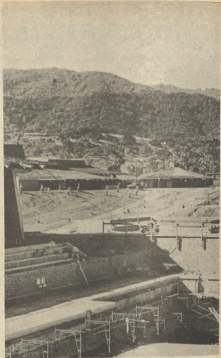
Foothill College is under construction in late spring, 1961. In the foreground is the Olympic pool as we look from the P.E. area across to the main campus. The Campus Center is at the right.
