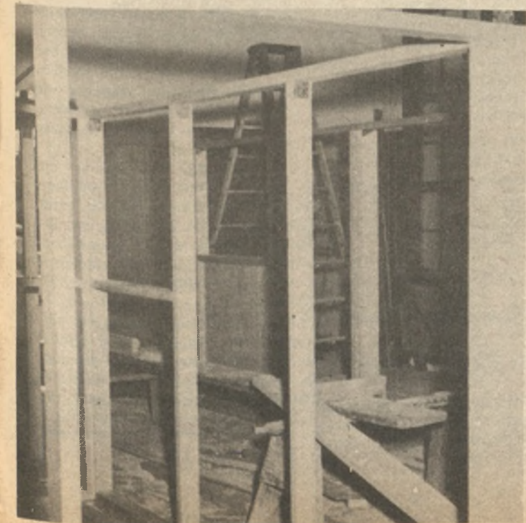
A counseling office under rehabilitation of the Old Highway School. The cost of rehabilitation went into the thousands of dollars.
