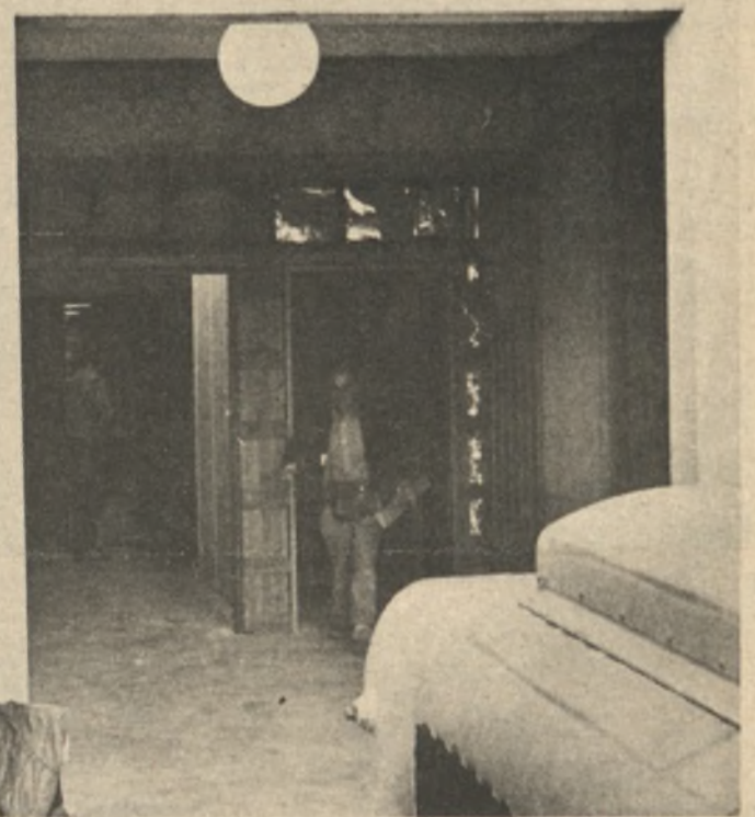
The construction now going on in the lower section of the Campus Center is scheduled to be complete in early April. The money for the building of these new offices came through student council on a loan to the Campus Center. Among the services these new offices will hold are: an enlarged Cop Shop, Placement Center offices, Financial Aids offices, and Multi-Cultural offices.
