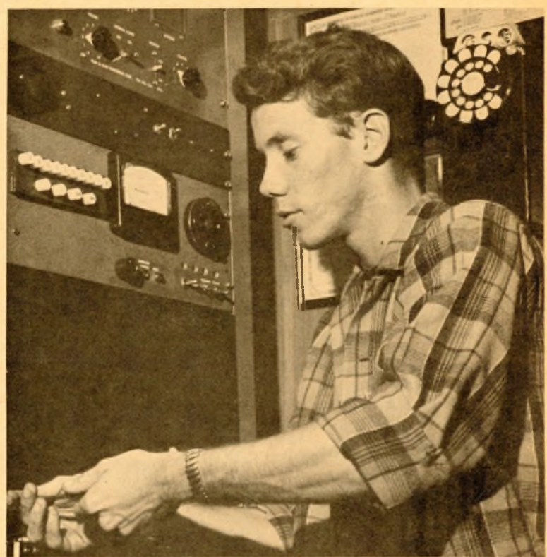
Jerry Bell, chief engineer, makes a last minute check on a portion of the transmitting unit.
