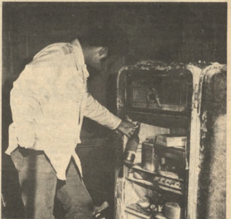
Ebe Hunter, ethnic studies instructor, surveys some of the damage caused by a raging fire which destroyed his home and most of his personal property. Fortunately, neither Hunter, his expectant wife, nor their little girl were hurt.
