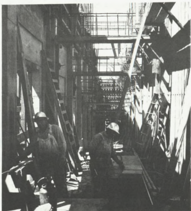
After being given a 70-day delay because of heavy March and April rains, workmen continue construction of the auditorium. When completed in 1970, the auditorium will be the largest between San Francisco and Los Angeles. (La Voz photo by Ken Jeffries)
