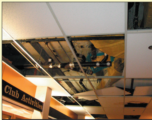
Removed ceiling panels outside of the Student Council Chambers as they appeared on Thursday.
