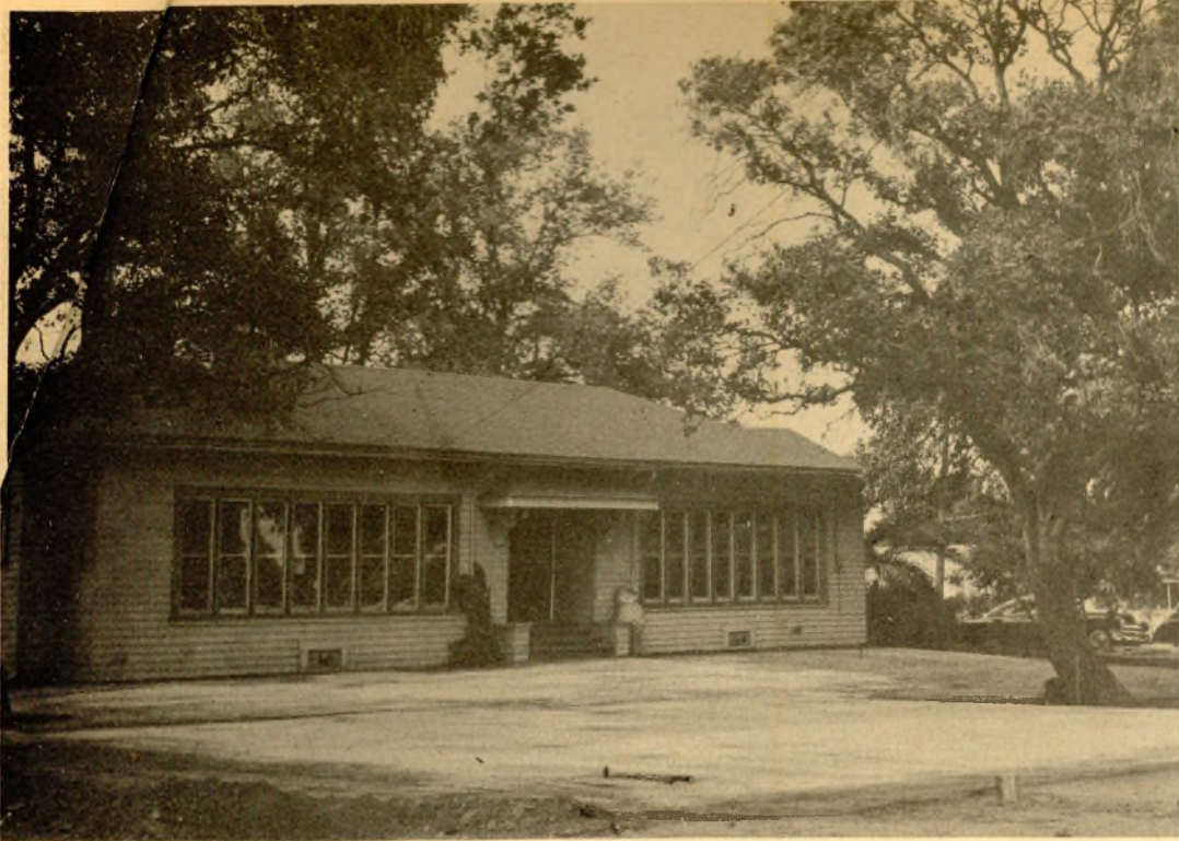
THE GROUNDWORK, THE OAKS, AND THE OWL. Short months ago only these elements were visible to the Foothill student. Construction had just begun on the most modern building on Foothill's campus. Behind the foundation and the owl lies the old building used expressively for a storage room for the bookstore. Now this building is hidden behind its new sister the student union.
