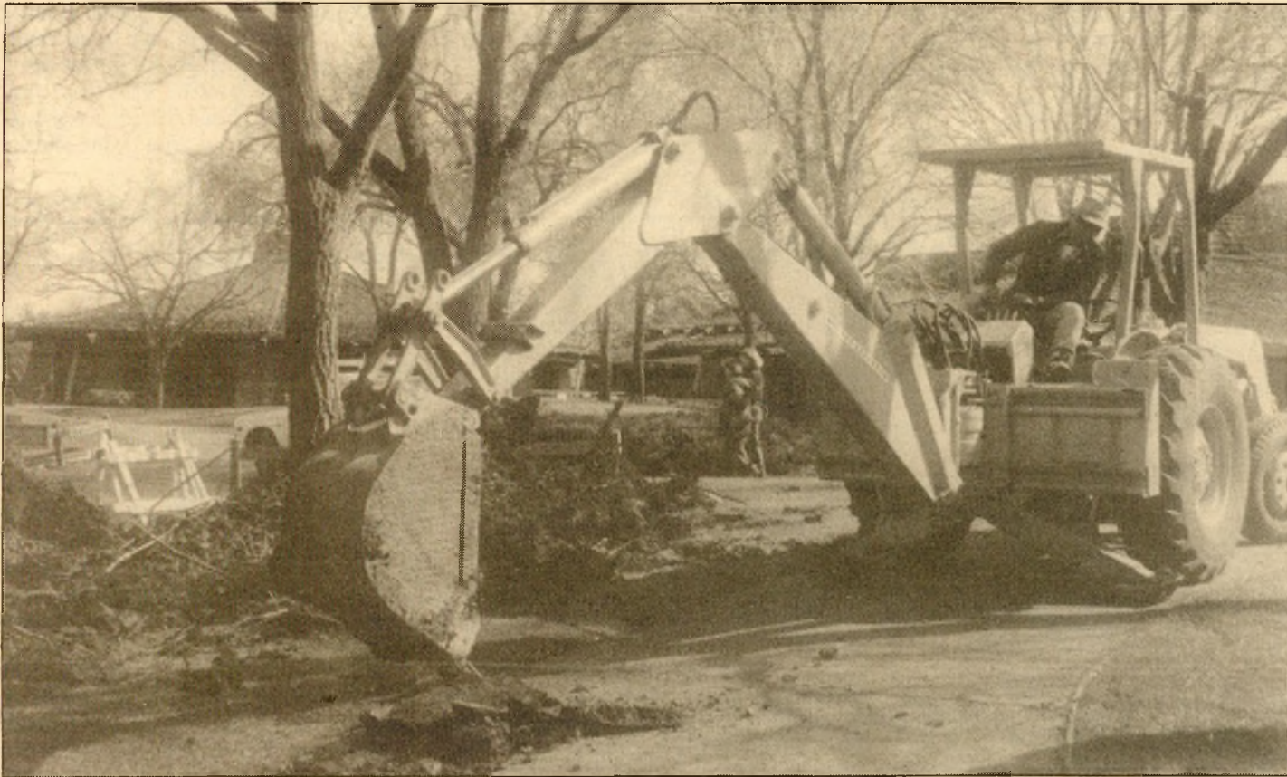
Back-hoe operator Joe Indalecio maneuvers his machine in front of the Foothill Administration Building. Construction work is underway to expand Foothill's KFJC (89.7 FM) radio station facilities on campus.
