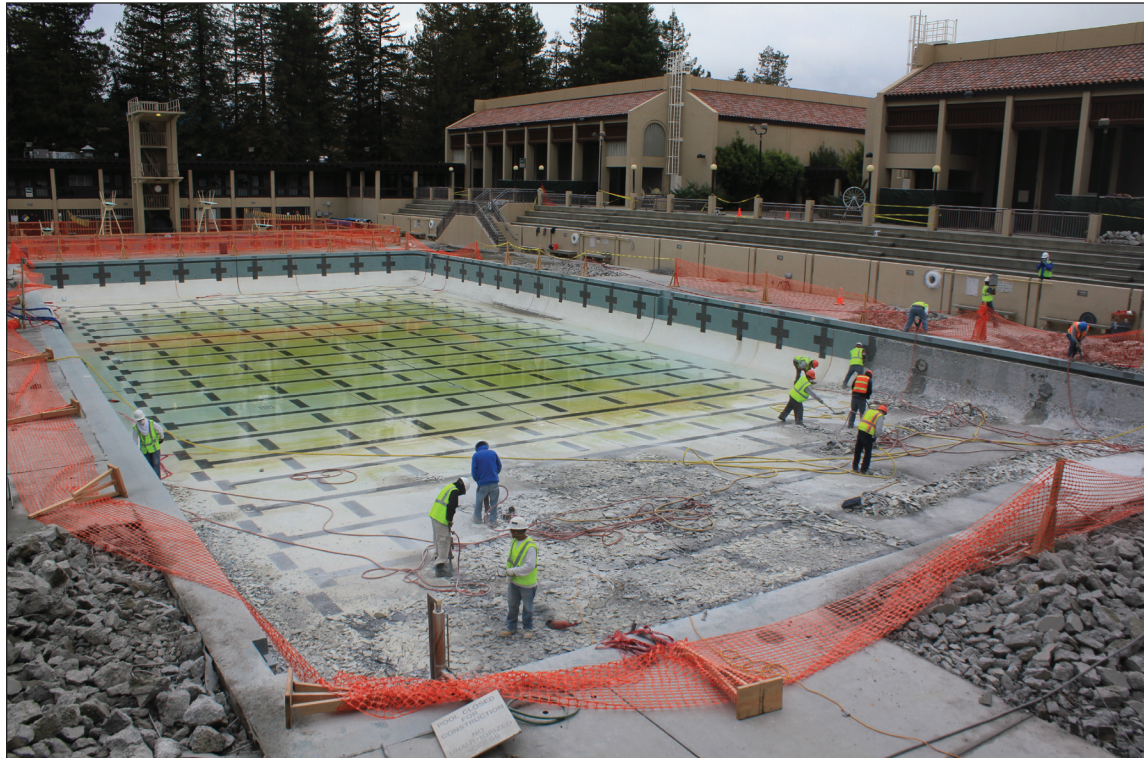
EMPTY POOL - A construction crew begins removing old tile and concrete from the bottom of De Anza's large pool. Both pools will remain closed during winter quarter as crews work to replace aging and damaged materials.
