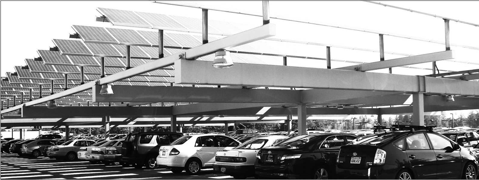
SITE [MOSTLY] UNSEEN - One of the many solar panels on top of Stelling parking structure helps supply energy and keeps cars cool.
