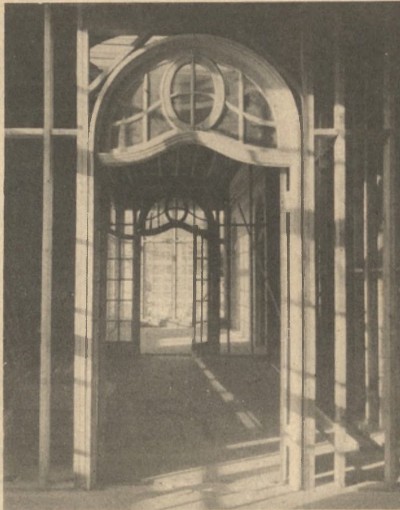
This room in the Trianon will eventually be the library. Photo by Joan Glelow
