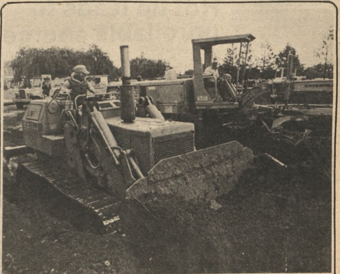
La Voz photographer Howard Lipin caught this jumble of earth-moving machinery Monday at the construction site of the new classroom building. The building, scheduled for completion early next year, will house several classrooms, as well as lecture halls and seminar rooms.
