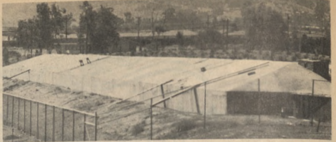
Construction of De Anza's new $363,000 pistol range begins. Located near the athletic field, it is scheduled for completion in June, 1969. The range will be used for law enforcement and recreational purposes. (La Voz photo by Rick Morgante)
