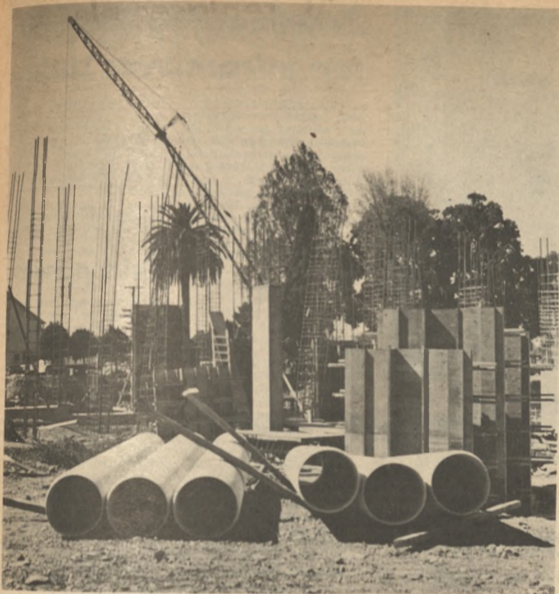
Construction has begun on De Anza College's 2600-seat auditorium. Completion of the theatre within the next three years will bring to the Peninsula community major Broadway road shows,
