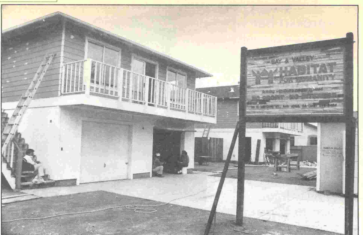
Above : One of the houses that is being built with volunteer labor and donated materials. Top right : David Grandos paints the window frames of the house that he is going to receive.
