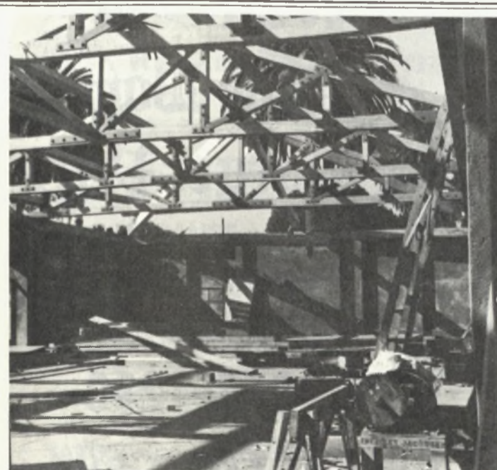
Construction is running on schedule for the Bookstore-coffee-shop, formerly the old winery.
