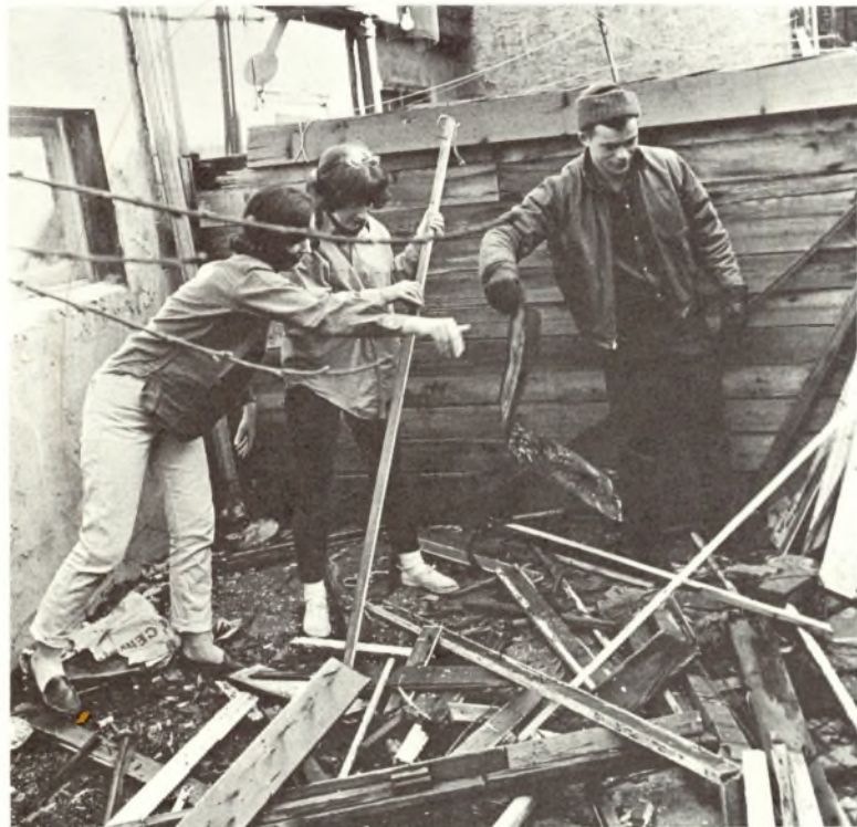
AS AN EXAMPLE to the rest of the neighborhood, VISTA Volunteers in west side Philadelphia cleaned up, repaired, and nearly rebuilt a dilapidated row house which will serve the girl volunteers as living quarters. Clearing debris are Mary Sullivan, University of Massachusetts graduate; Mearan Brown, who attended San Jose State College, and Frank Rubright of Alma College.
