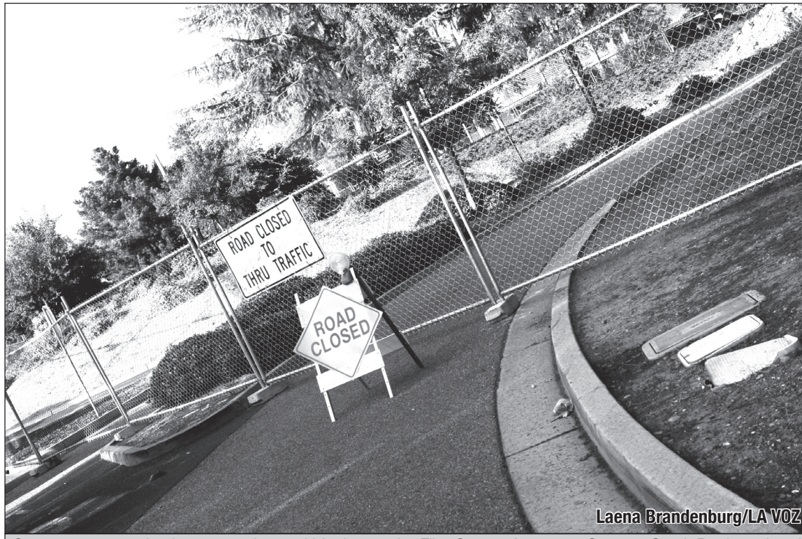
Campus construction has created a road block near the Flint Center. Access to Stevens Creek Boulevard and Highway 85 entrance is now blocked, adding to the existing traffic jam following class ending times.
