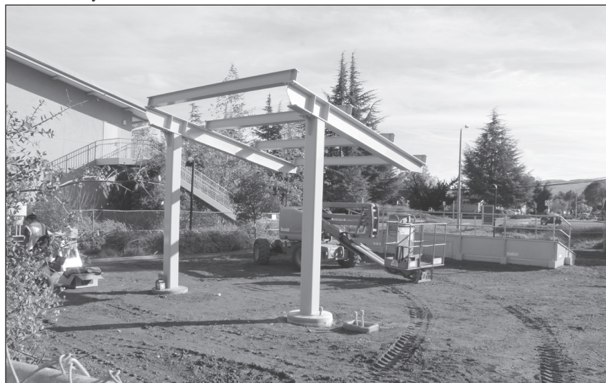
HERE COMES THE SUN - New solar panels are being installed outside the Kirsch Center ready to interact with the center's Solar Education and Demonstration Lab.
