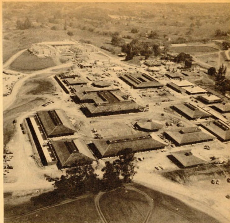
OWL'S EYE VIEW—This aerial view of the new El Monte Campus shows the plant 63 per cent complete. The 10.4 million dollar campus is being constructed on 122 rolling acres on El Monte Ave. Building groups include the P.E. department, upper left; fine arts and auditorium, upper right; the library in center; the administration building which is the smaller structure to the upper right of the library; and the campus center, between the administration building and the P.E. plant. (photo by Air Photo-Co.)
