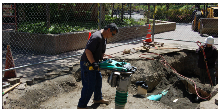
Andy Gurrola and Tim Mechikoff work around the pipes they are repairing by the Campus Center on April 9.
