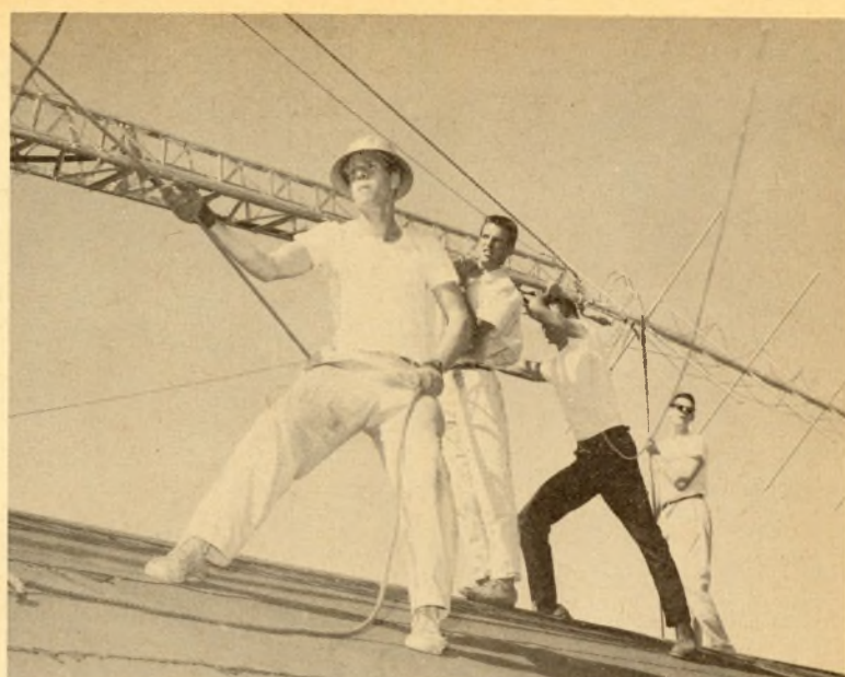
UP SHE GOES—Bob Ballou, pulling rope, begins installing radio antenna. Working behind him are Jim Fernbaugh, Nathan Ballard, and Roger Murray.
