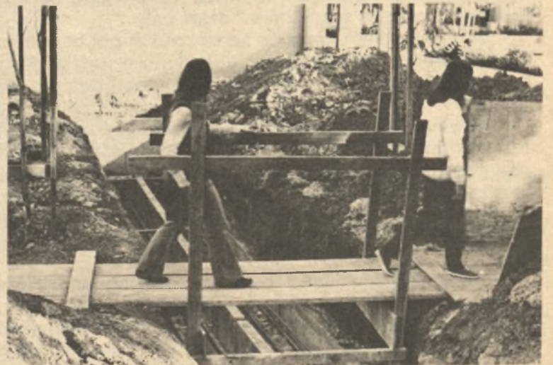
An unsteady bridge used by students who have classes surrounding the Fine Arts Division will be there for "at least another month," according to Inspector Walter Egnew. The bridge is over a ditch where heating and cooling pipes for the auditorium will be placed.
