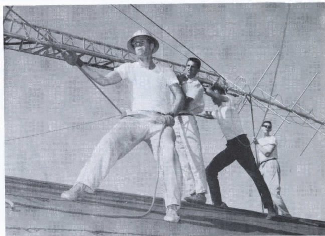
BIG LIFT BEGINS —The KFJC antenna at Foothill College began its climb to an upright position with this effort. Students, friends and the faculty advisor to the FM station worked together three consecutive weekends to place the transmitting antenna on the building's roof. Bob Ballou, pulling the rope, is the student manager of KFJC. Working behind him are: left to right—Jim Fernbaugh, Nathan Ballard and Roger Murray. The station will go on the air sometime this month.
