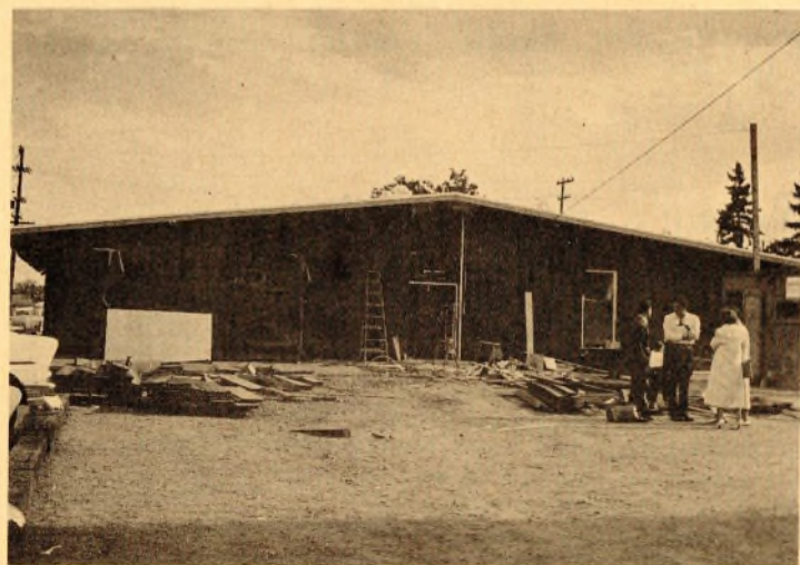
TEAM SPORTS LOCKER ROOMS—It is possible that the men and women physical education classes will be using these facilities by Nov. 26, barring any further unforeseen delays in construction.—(Photo by Len Walker)
